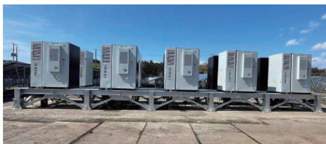
Renon DC ECube 215kWh*
