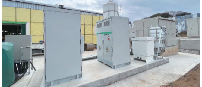
Renon DC ECube 157 kWh
