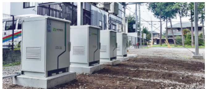
Renon DC ECube 15 kWh
