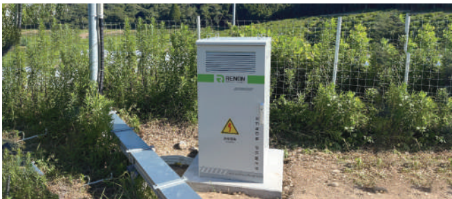
Renon DC ECube 38 kWh
