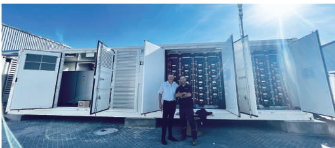
Renon Estation 744 kWh
